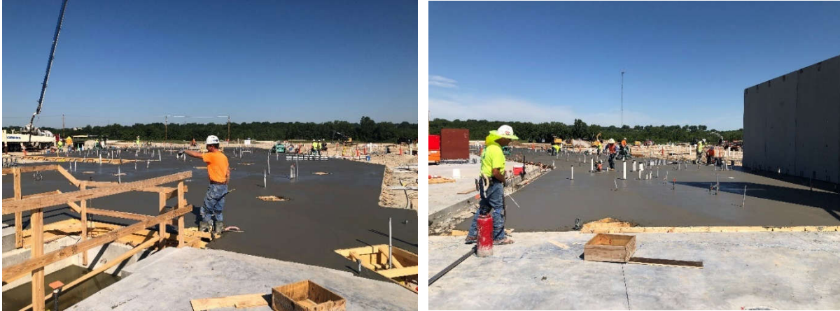
Pictured above: additional slab on grade pours expanding the building footprint that is constructed.
