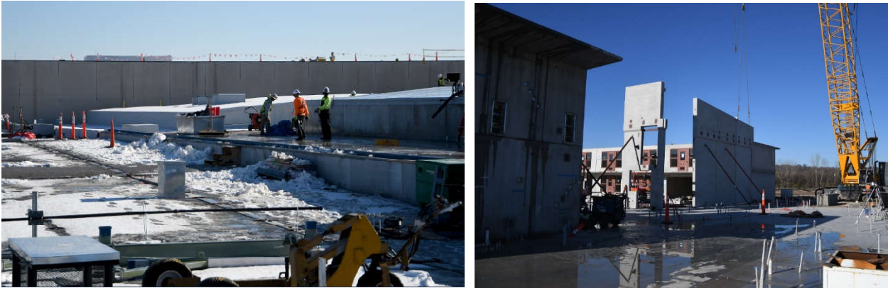
Above: Construction continues throughout winter conditions whenever possible to maintain the schedule.
