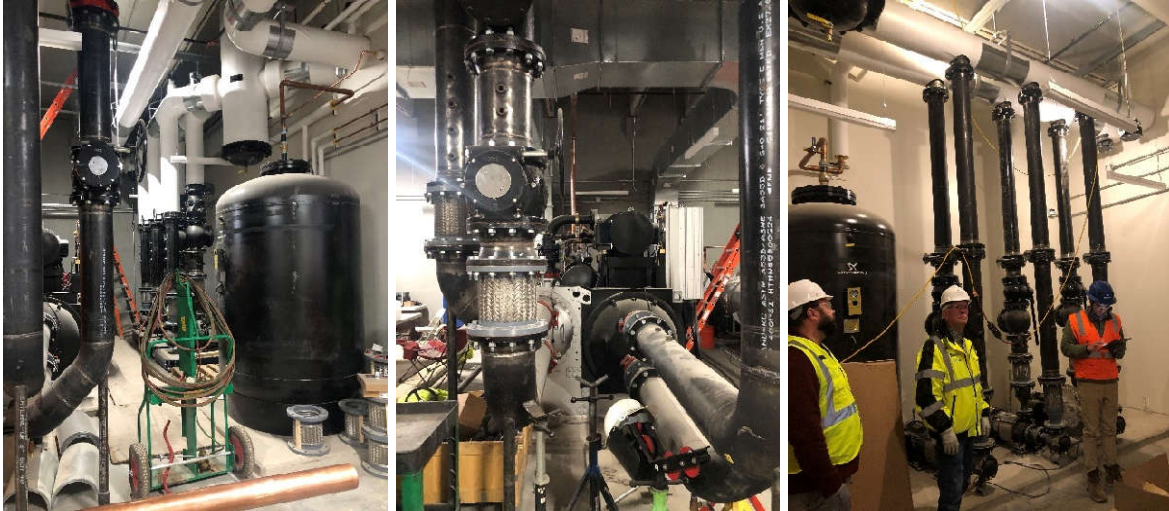
Above: Central Utility Plant equipment installed and County staff touring for a deeper understanding of the building systems and their operation.
