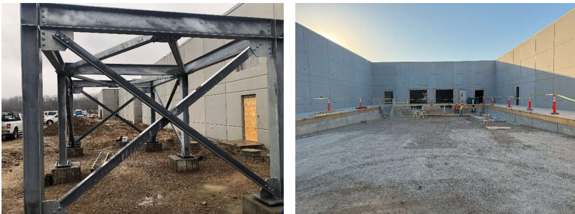
Above: Cooling tower steel erection behind the Central Utility Plant and the loading dock area.
